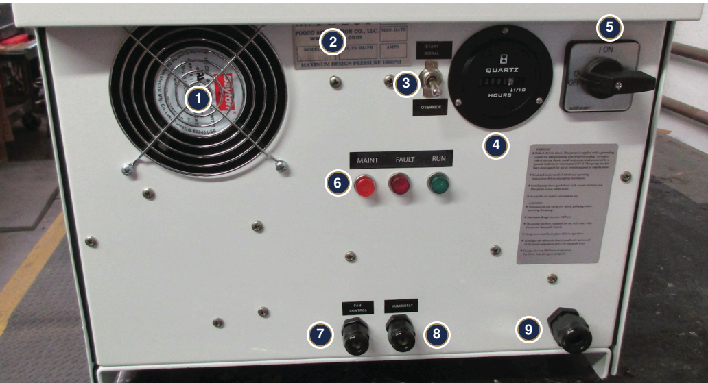
Figure 2 — Electrical exterior end of the Pump Station enclosure.
