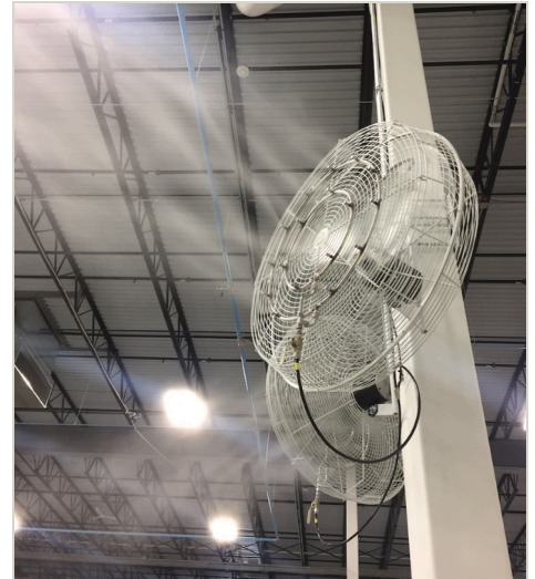
Figure 1 — FanMist 36" fan with mist ring, fed at 1000-psi from the Pump Station.
