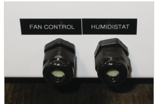
Figure 6 — Exterior strain reliefs, marked FAN CONTROL and HUMIDISTAT.
