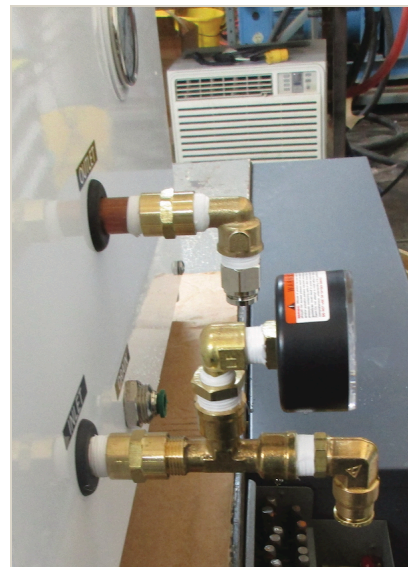
Figure 3 — Side view, water facilities end, showing the brass fitting assemblies stepping out from the enclosure wall.
