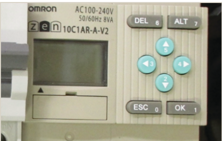
Figure 8 — Omron 10 I/O PLC on the electrical panel DIN rail.
