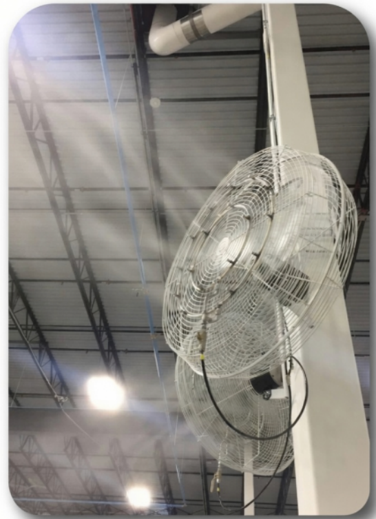
1000 psi High-Pressure Misting System with High-Velocity Fans
