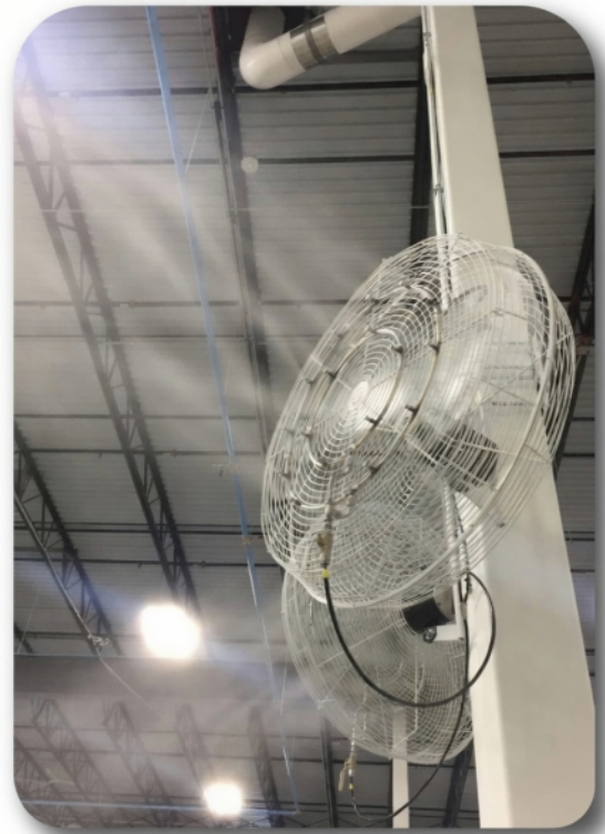
1000 psi High-Pressure Misting System with High-Velocity Fans
