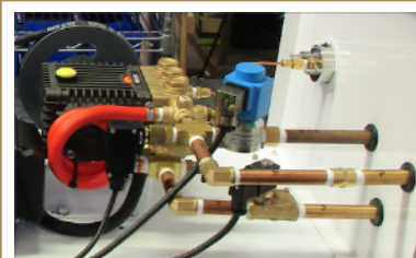
Fig. 10.3 EDV LOCATION Mounted on the Pump Output Line
