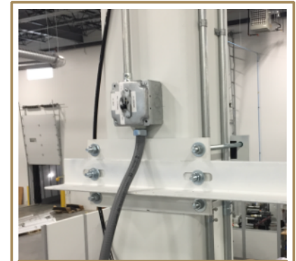
Fig. 5.5 LOCAL DISCONNECT SWITCH Mounted to Structural Beam
