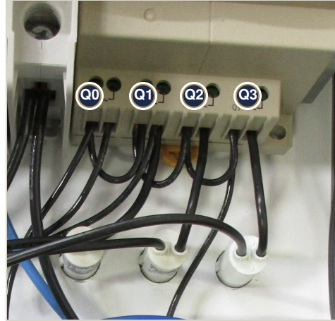
Figure 2 — PLC output relays Q0 – Q3, shown before conversion.
