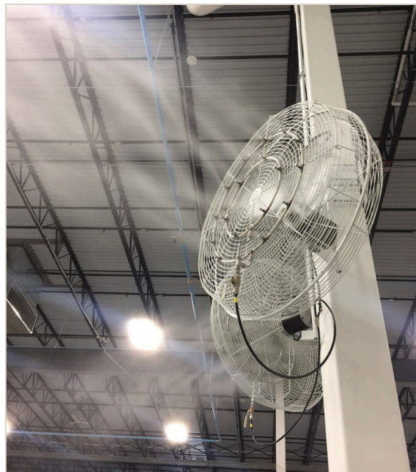
A FanMist 36" fan and mist ring delivering its plume into the warm ceiling zone.
